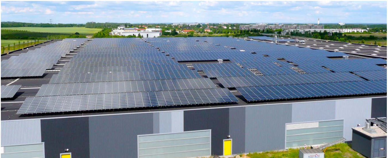
2.9 MW Rooftop PV Installation at First Solar's Recycling Facility in Frankfurt Oder, Germany.
