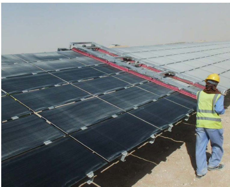
First Solar Manual Dry Brush Trolley at the 13MW DEWA solar PV power plant in Seih Al Dahal, United Arab Emirates
