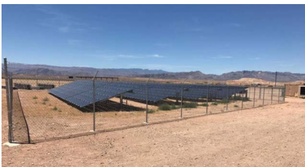
15kW Veterans Park Solar System
