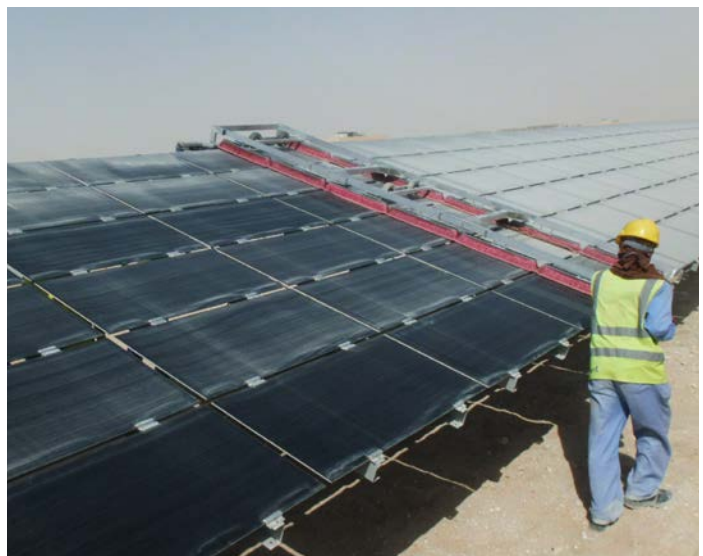
First Solar Manual Dry Brush Trolley at the 13MW DEWA solar PV power plant in Seih Al Dahal, United Arab Emirates
